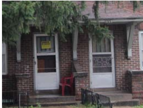
The unit on the left has been tagged as unsafe.
