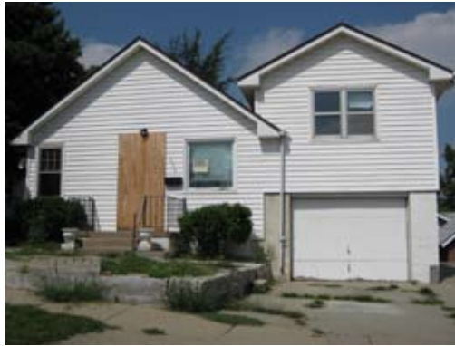
This house has been deemed Unfit / Unsafe by City inspectors.
