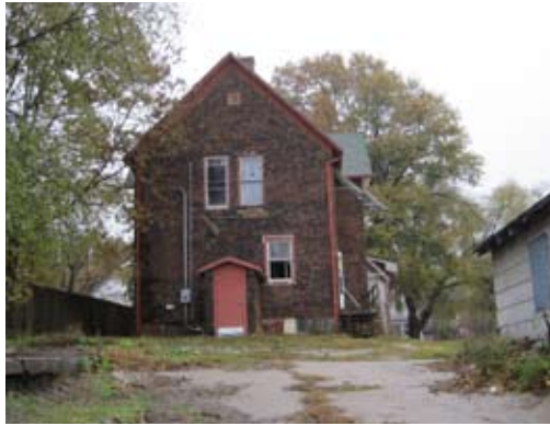
Houses with serious code violations should be targeted for expedited demolition or renovation.
