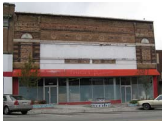
South 24th Street storefront in need of restoration.
